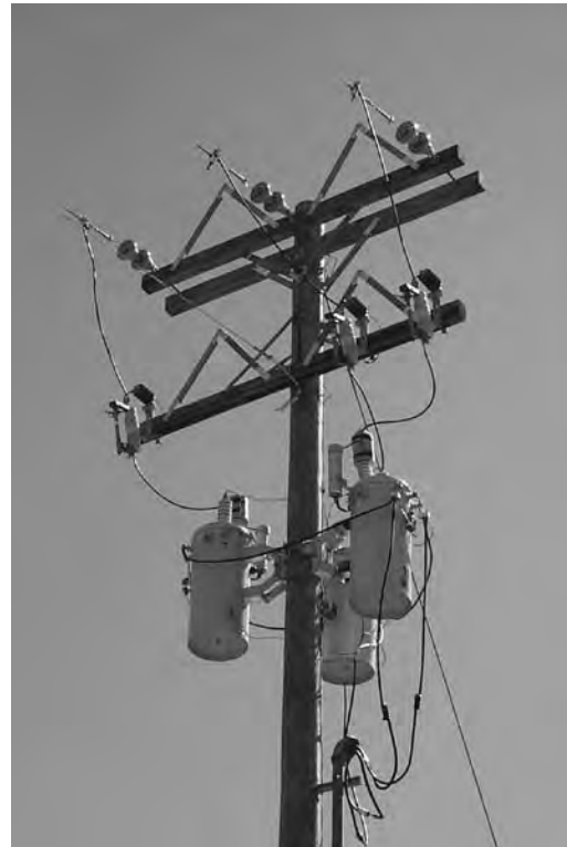
Protective equipment has been installed on this power pole to discourage raptors from roosting, perching, or nesting.
